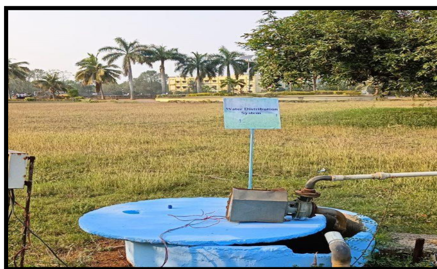
Water distribution unit in MIST Campus
